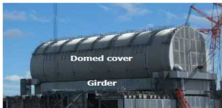
The domed cover on Unit 3 reactor building (As of March 2018) (Photo provided by TEPCO)
