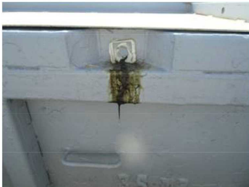
Leakage from tank No. 1-3
