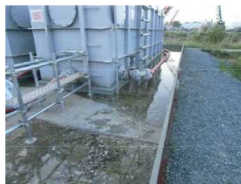
Rainwater accumulated in the dike
