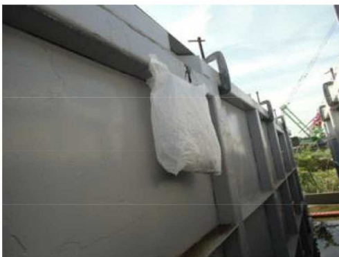
Vinyl bag attached to hold leaking water
