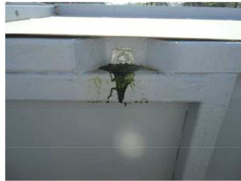
Leakage from tank No. 1-5
