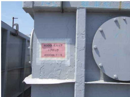
Photograph 1 Leaking notch tank
