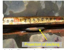
Back side of bottom plate at leakage path area before disassembling (Sling bottom plate A and B straight up and check)
